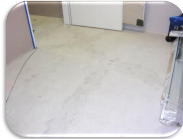
Cracked cement floors
